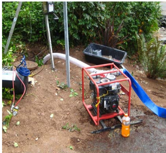
Figure 5-15. Bypass Pumping Setup.
