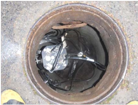
Figure 2-7. Flow Meter Data Logger.
