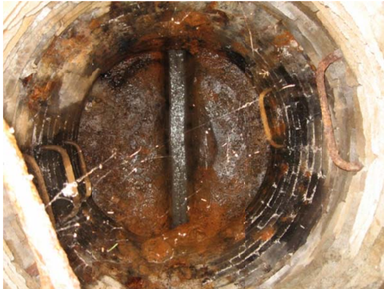
Figure 5-13. Leaky Concrete Block Maintenance Hole.
