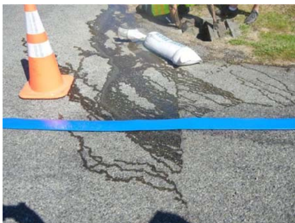
Figure 6-14. S1 Leaking Through Pavement.
