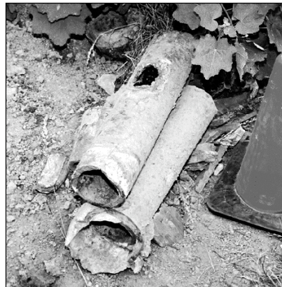
Example of the condition of laterals that were relined in Tacoma, Washington.
